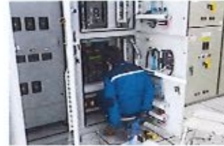
KCC Factory (Anseong)
